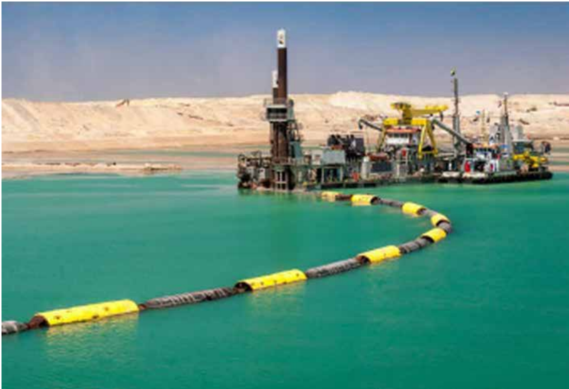
Surface floating pipeline
