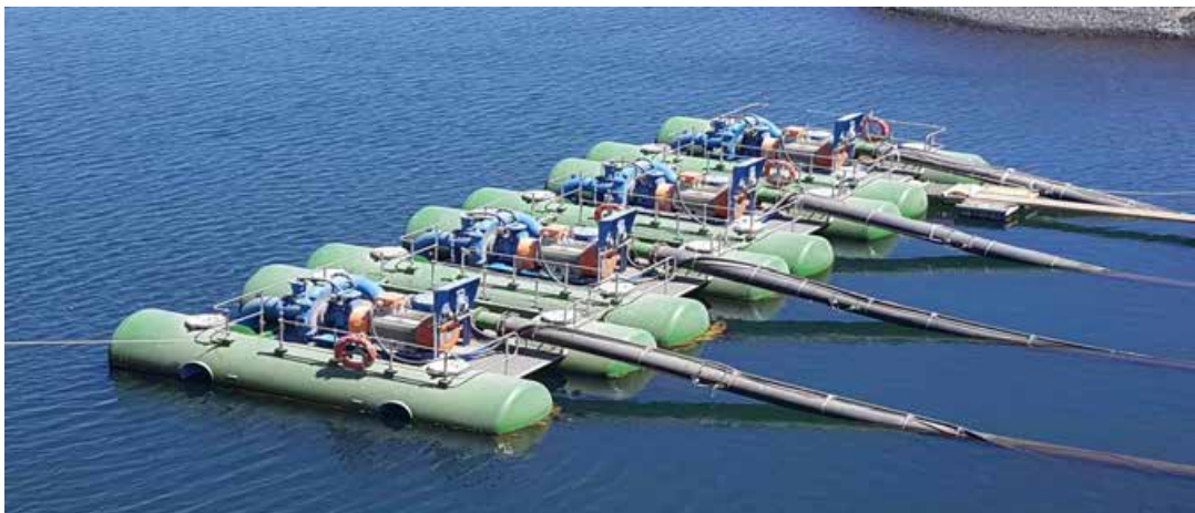
Wastewater transportation with floating pontoon pipeline systems
